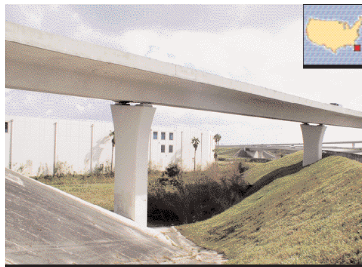
The Freyssinet teams inspected 10,000 m of internal bonded PT cables and 628 anchor heads.
