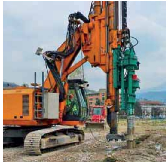
MENARD used its expertise and tools to carry out a novel soil remediation operation in Voiron in southeastern France.
