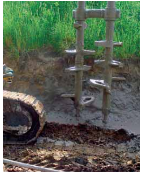
ENVIRONMENT. Menard used the soil mixing technique, carried out with a twin auger, to remediate a chlorine-contaminated brownfield site in southeastern France.
