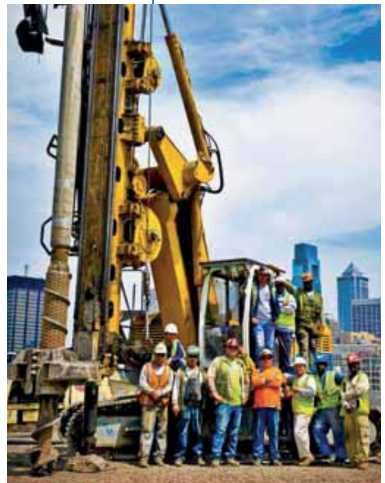
ON THE PENN PARK PROJECT , the alternative solutions designed and implemented by Menard, Nicholson and Reinforced Earth Company saved the customer several million dollars.
