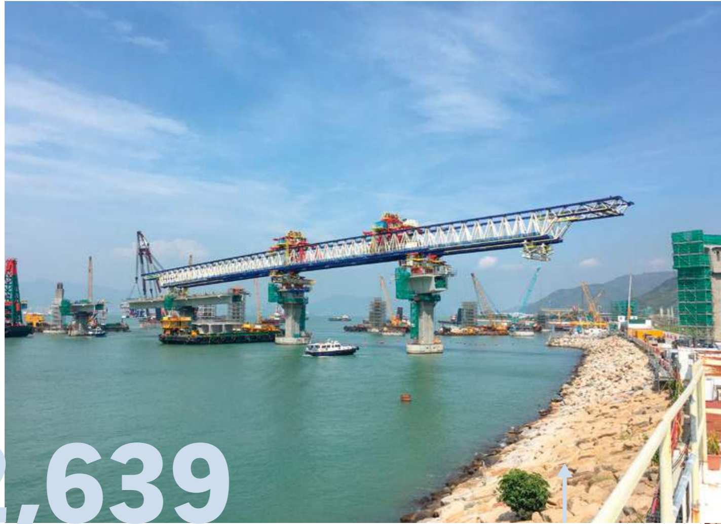
TMCLK viaduct Tuen Mun - Chek Lap Kok, Hong Kong
