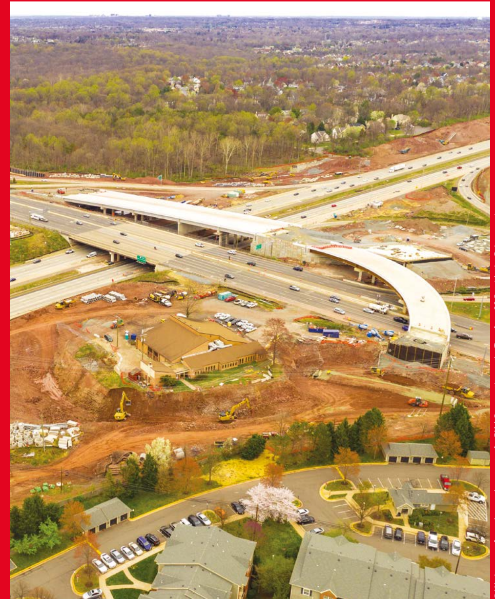
© Work was performed as a subcontractor for FAM Construction on the Transform 66 Outside the Beltway project
